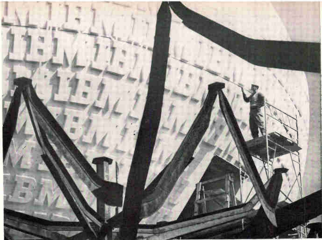
Resembling a huge Easter egg, the IBM ovoid contains a 500-seat theater. The structure carries the letters IBM almost 1,000 times.
