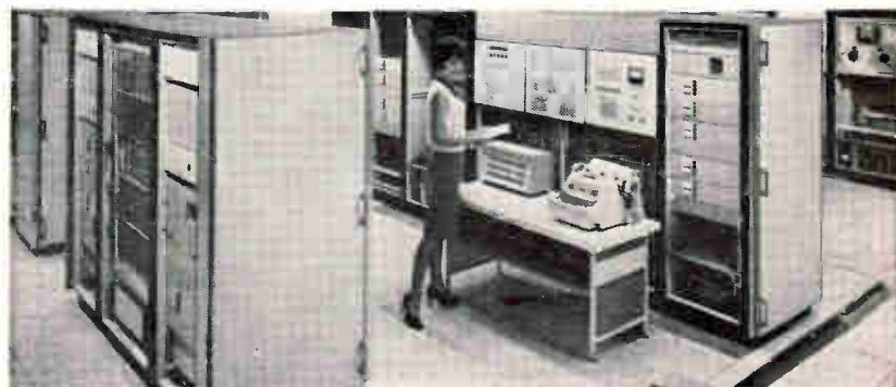
THIS IS FIRST PHOTO released for publication of data-processing system that Librascope is building for Air Force's 473L command and control system. System includes mass-memory disk file (left), central computer (center) and magnetic tape consoles (left and right). This system is to be used in the Pentagon
