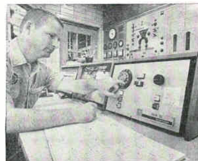
ON-LINE controller for Gulf States Paper plant is Westinghouse Prodac 580 computer. It runs 350-ton-a-day pulp digester
