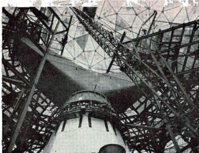
LATEST PHOTO of Haystack antenna being constructed under radome. In an operational orbital scatter system, this facility could provide many voice channels
