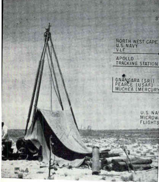
DRILLING RIG probes shimmering white limestone salt flat, to insure there will be no caverns under tower foundations at Navy's vlf station
