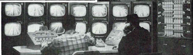
TELEVISION MONITORING and traffic-control center for the Detroit freeway with confirmation panel at right
