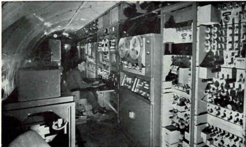
Flying television station carries six tons of telecasting equipment. Facilities installed by Westinghouse include master control panel, two video tape recorders, two high-powered transmitters and a vidicon camera to transmit announcements and station identification
