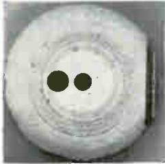
Two small holes inspected at bottom of 2½" deep hole.
