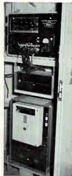
Clock, control unit, and recorder mounted in the Gyro Room of the Mormacpride's Bridge Deck.
