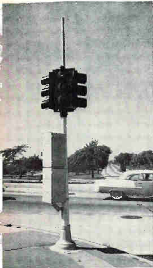
Signal pole houses radio receiver and control gear, responds to signals broadcast from central control location
