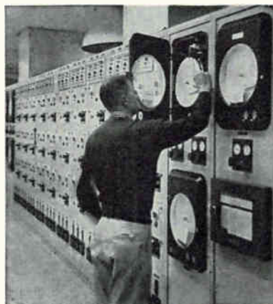
Electronic temperature controllers made by Hagan Chemicals & Controls help produce fiber glass yarn
