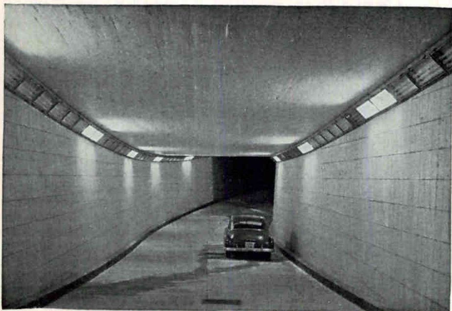
Automatic light control continuously adjusts tunnel illumination so that it equals the ambient light outside, thereby preventing automobile drivers from being temporarily blinded
