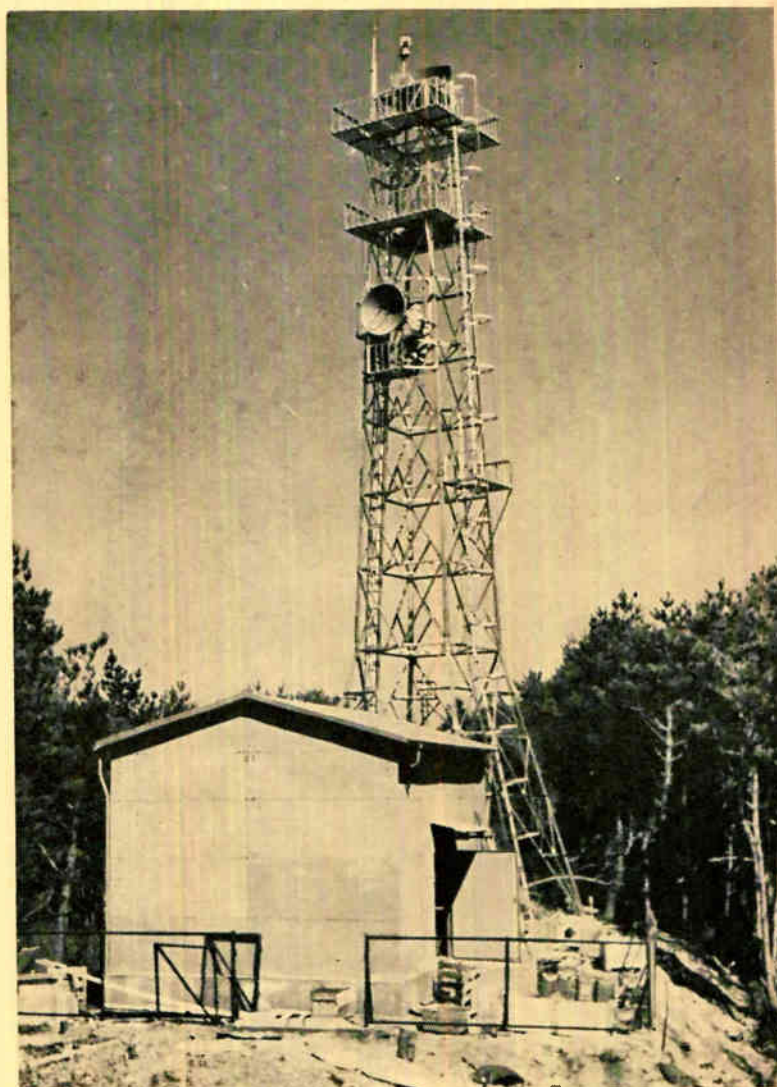
This 12,000-Mc link built by NEC is used for remote control of a lighthouse in Hokkaido
