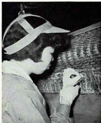
Tatsuko performs an intricate series of wiring jobs on automatic switchboard assembly line
