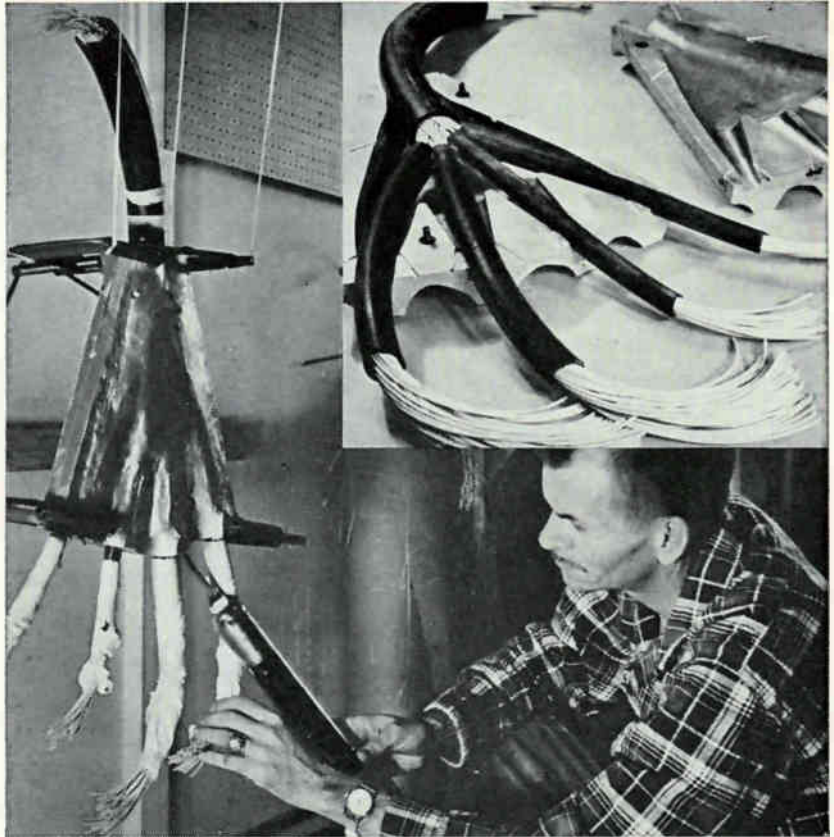
Molding a junction. Compound is injected from bottom to top to permit air to escape. Note direction of threaded ports in mold (insert)
