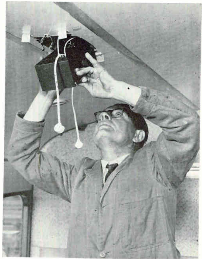
One inverter for each lamp is installed in ceiling
