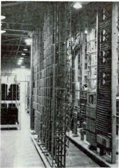
All messages pass through the distributing frame in the cable terminal building in Thule, Greenland, where they are terminated and rechanneled to other communications facilities
