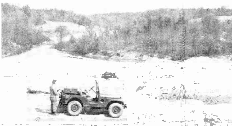
Operation of bulldozers in hazardous areas is accomplished remotely with a standard Signal Corps radio. The system, performing 13 distinct functions to control the bulldozer, was developed at the U. S. Army Engineer Research & Development Laboratories, Fort Belvoir, Va.
