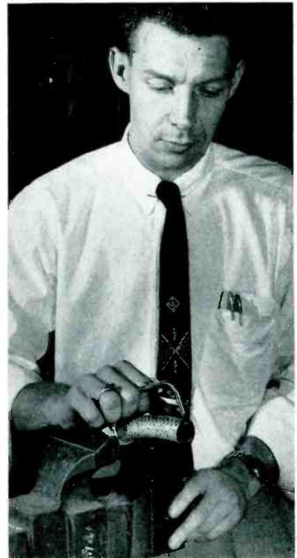
Slitting cable armor with special knife while cable is held in vise. Cushioning material prevents vise jaws from damaging cable
