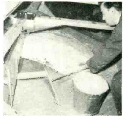
Burlap dipped in plaster and laid on wire mesh provides base for plaster
