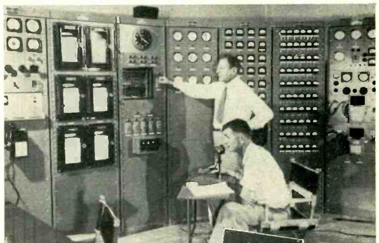
The complex instrument panel in the control room of Control Point, Yucca Pass, Nevada Proving Grounds . . . The Precision Timers on the fourth and seventh sections are by Standard.
