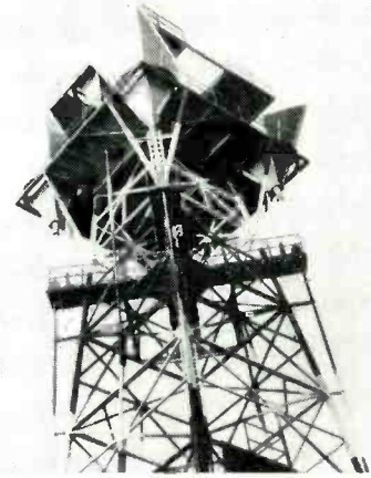
FIG. 2—New type of microwave antennas installed on tower near Terrell, Texas. Single antenna can handle 15,000 telephone conversations and 10 tv programs simultaneously
