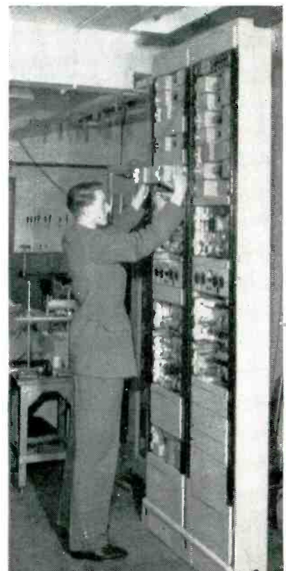
Relay station equipment undergoing tests prior to installation in the Alps
