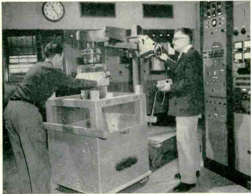
Operating engineers Saul Osias and Eric Potts prepare to replace final-amplifier tube weighing 250 pounds using motor-driven hoist on dolly. Auxillary 10-kw transmitter is in background. Racks at right hold measurement and control equipment shown in separate photograph at left
