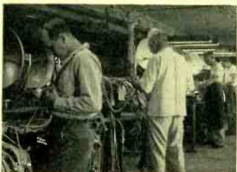
Control and Junction Box Assembly and Inspection.
