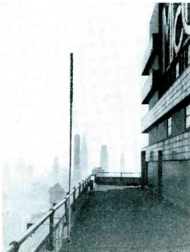
Colinear array installed on roof of McGraw-Hill Building for long-distance tests of citizens band coverage
