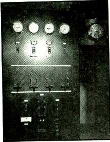
An inter-office distribution panel for the precision clock control circuits
