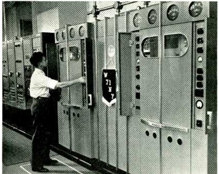
A new 10,000 watt transmitter of W71NY, frequency modulation station of WOR, N. Y., is now on a full-day broadcast schedule
