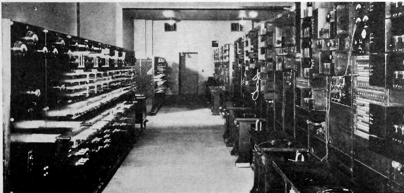
Amplifier room of a modern sound studio. Amplifier equipment for eight recording channels is shown at right with power control panels at left. Estimated cost of the total electrical equipment involved, $1,000,000.
