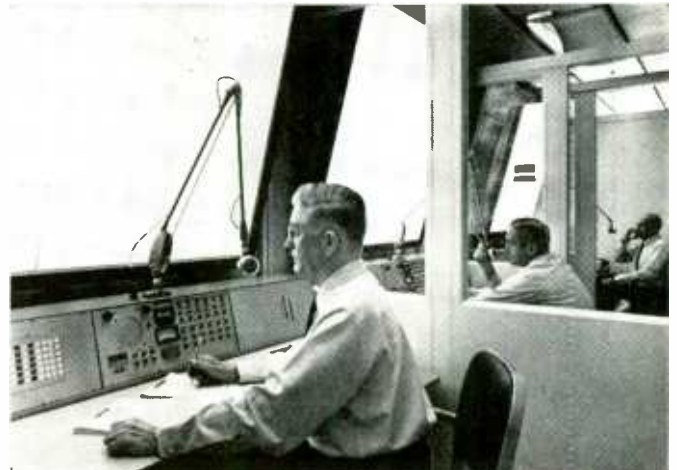
Control center for new bus radio system employs 19 radio dispatchers for the radio base stations. Telephone lines are used to connect dispatchers' consoles to the stations that are located in Transit Authority garages in the city's five boroughs.
