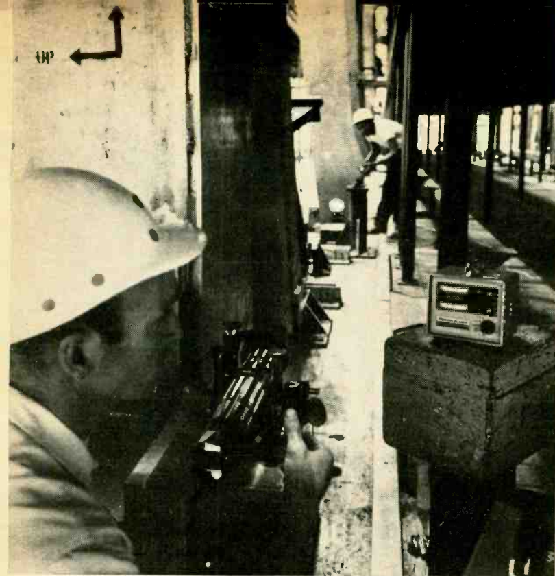
The straight, narrow beam of laser light is used to align tool jigs for the Boeing 747 transport. Accuracy is 0.01" in 200 ft.
