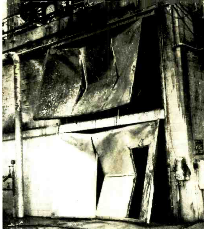
The Atlas Centaur explosion (see color photograph on the cover) caused this amount of damage to the doors on the launching pad.
