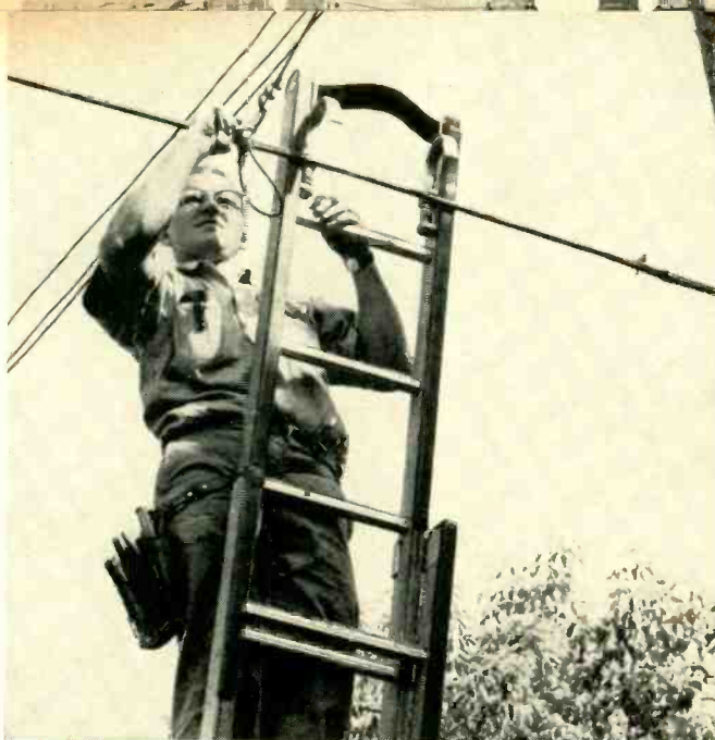
Technician installing pressure tap on distribution line for housedrop. Note strain-relief arrangement used here.
