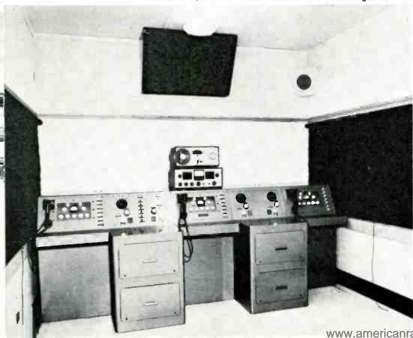
Multi-channel sound system installed in a modern high school.
