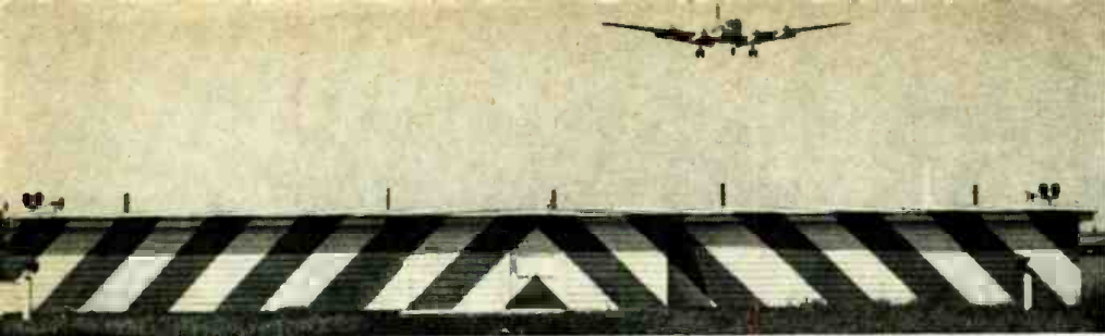
ILS localizer transmitter shack. The localizer array inside the building is an 8-antenna linear array. Two antennas, which are placed close together in the center, radiate the modulated carrier signal, and the other six loops are placed symmetrically on either side to form the necessary horizontal localizer course.
