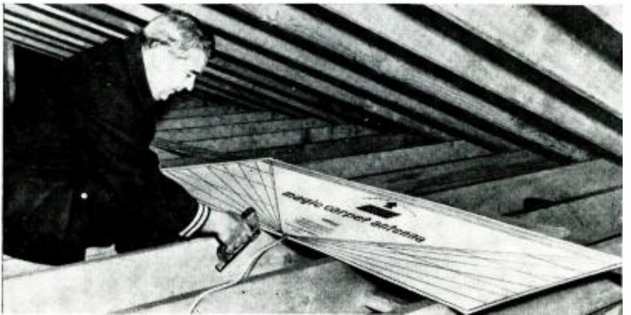
Permanent installation: a "Magic Carpet" being stapled to joists in the attic.
