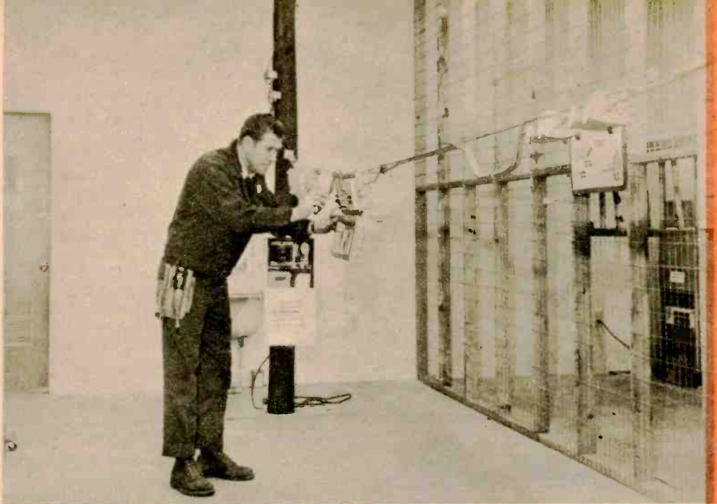
Some CATV companies go to great effort to train their men. This mock-up, with pole, cable and line amps, is at Tri-County Cable TV Co. in Salem, N.J. Set-up allows men to make tests in working system.
