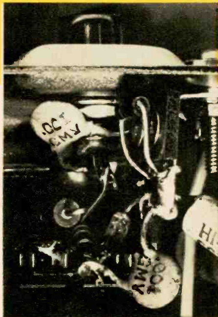
Fig. 1—Although solid-state CB rigs have next to nothing in the way of extra space, there's always a little near the output jack. Circuit at top is shown installed in the photo above.
