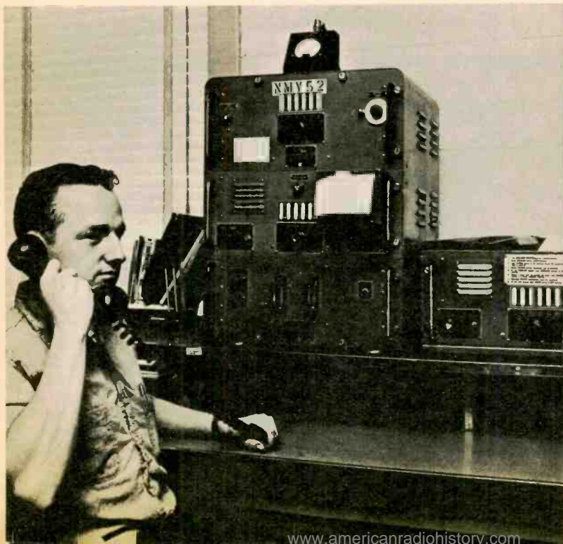
On shore, radio operators stand by in a round-the-clock watch, ready to relay distress calls from pleasure craft and fishing vessels anywhere in the New York/New Jersey coastal waters. Modern as the little rescue ship itself, the shoreside installation includes a teletype for speedy communication with other Coast Guard monitoring stations in the immediate area. Main Coast Guard center on shore is located on Sandy Hook, the tip of land which lies in front of entrance to New York Harbor.
