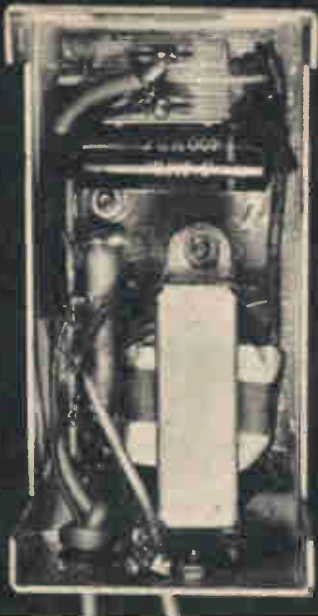
Components within the case are seen behind front cover. Transformer T is at lower right.
