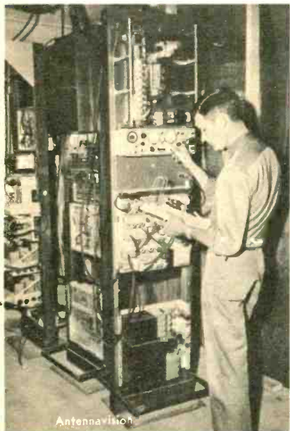
Microwave technician checks frequency tuning on receiver at master antenna site of a system that requires long distance relays.
