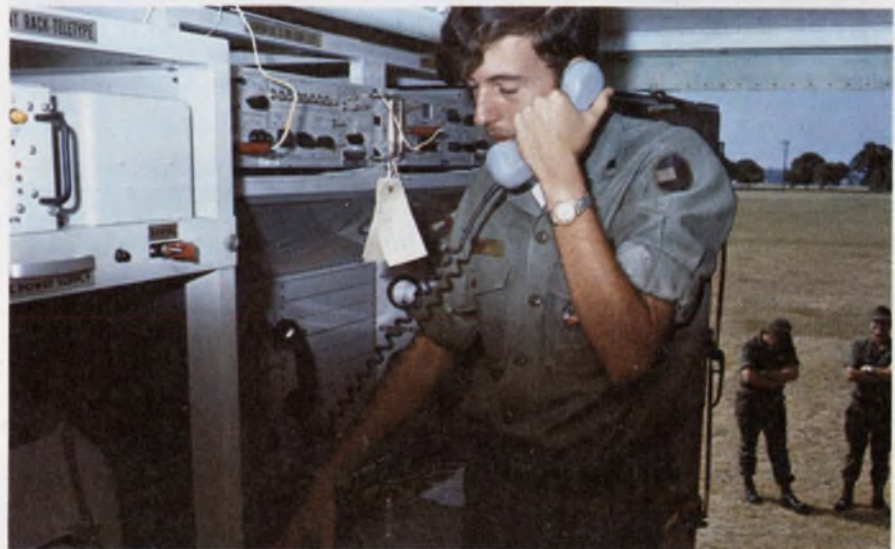
Technical Control Facility, AN/TSQ-84A, built by the Army, interconnects, monitors and tests up to 432 full duplex channels.
