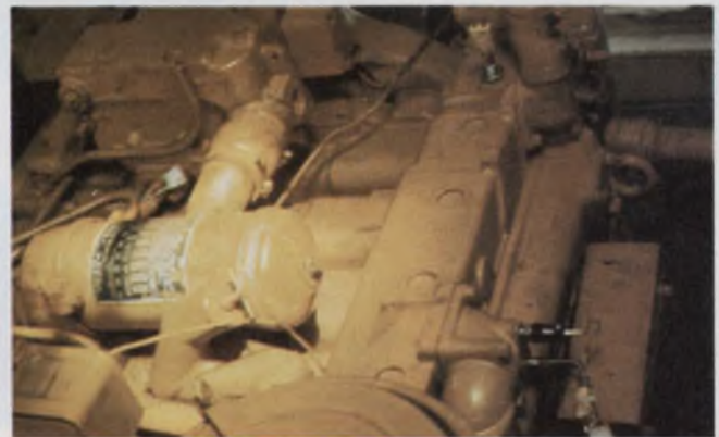
Microprocessors monitor marine-engine performance for maintenance and failure prevention. This diesel generator is watched by an Advanced Electronics Development Corp. system using gas, water and oil sensors.
