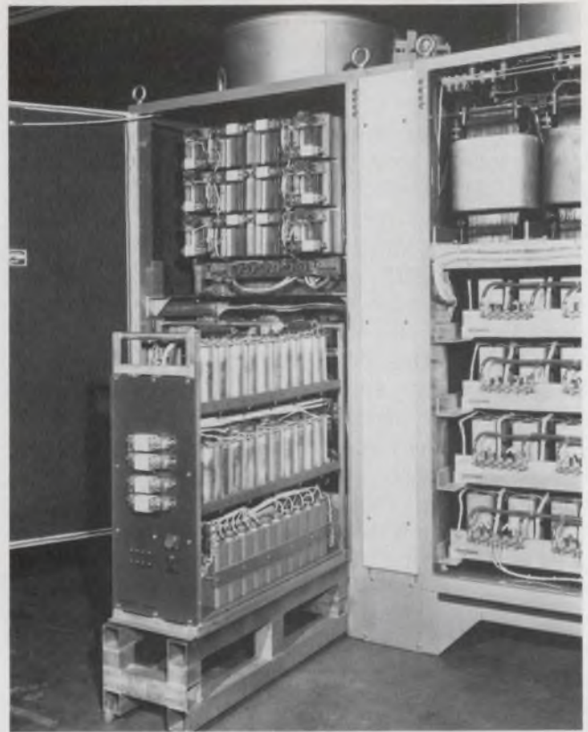
Massive power source on wheels: one of three Teledyne Inet inverter switching sections, mounted on rollers for maintenance convenience.
