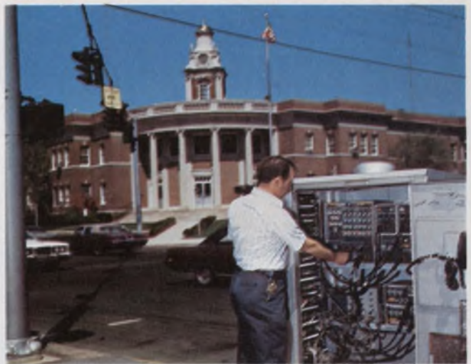
This traffic controller is a key element in a Connecticut system by Automatic Signal, Norwalk, that cut travel time by 45% through a high-traffic shopping district. Local intersection control is exercised by a CMOS microcomputer that talks to the system computer.
