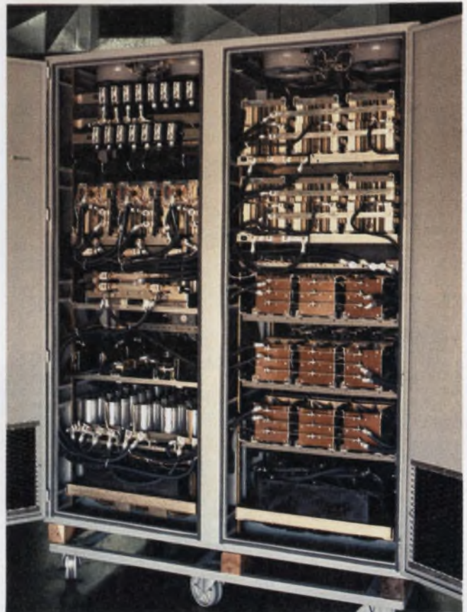
kVA UPS (left). The system includes a rectifier/charger, inverter and static and manual switches (right).
