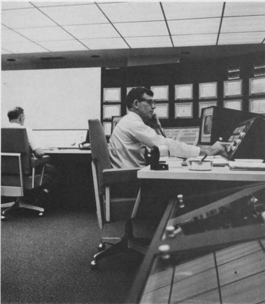
Electric utility control system built by Leeds & Northrup uses the company's Speedomax recorders on the wall to keep dispatchers posted on frequency and load conditions telemetered from key points.
