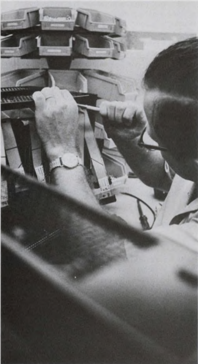
Advantages of flat flexible cable are apparent in this complex interconnection task—the wiring of an IBM computer mainframe.
