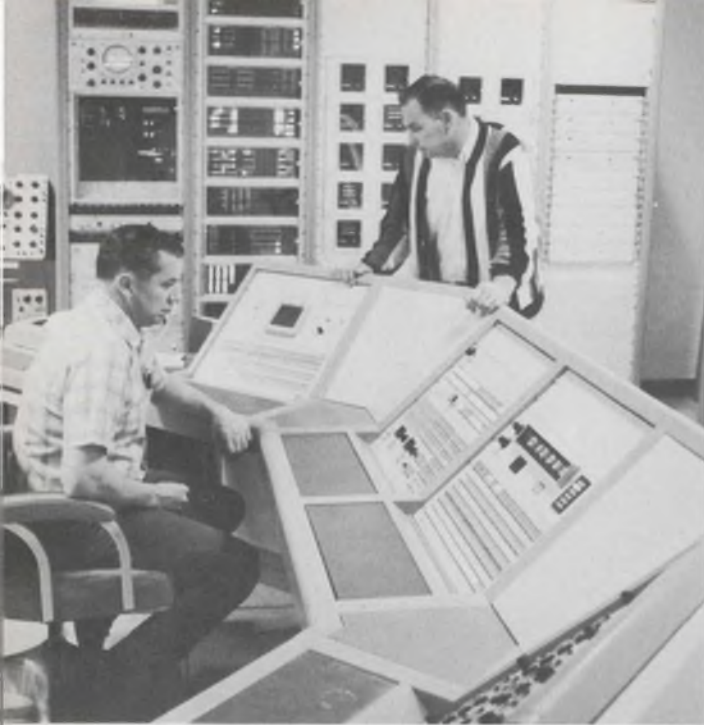
Tactical Acquisition and Data Control System being installed in the Flight Vision room tells radars where to acquire incoming planes.
