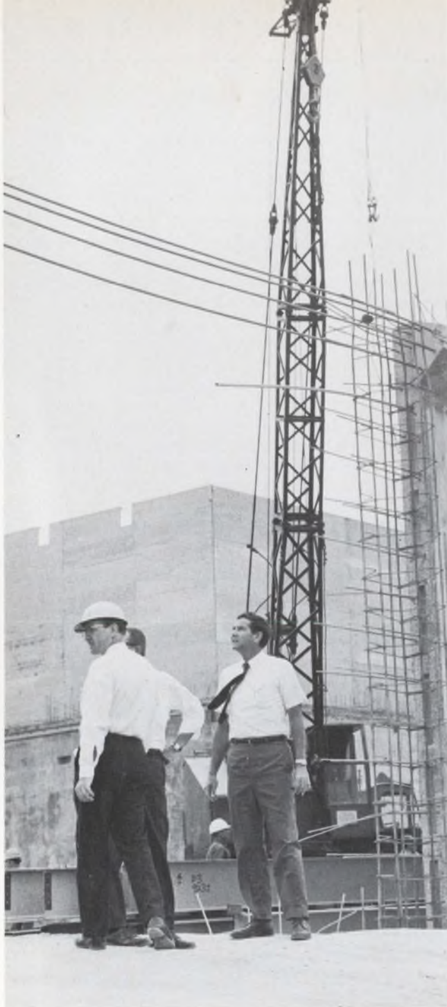
President Sporck surveys National's future corporate headquarters, a 115,000 square-foot plant under construction in Santa Clara, Calif.
