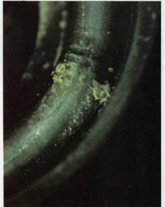
The entry of chemical agents caused a small section of the element to deteriorate. The resultant chemical action caused noisy performance.
