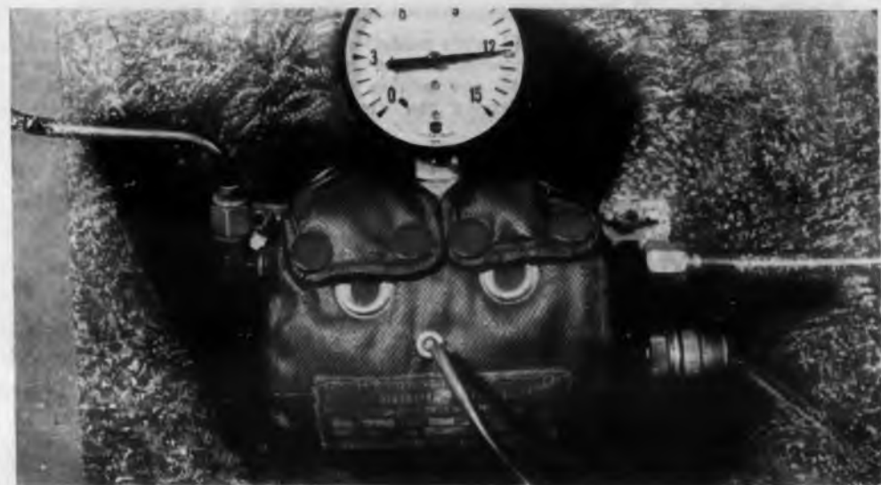
SPECIAL HEATING unit custom-designed and delivered by G.E. in 5 days enables stock valve to function properly, saves customer time, money.
