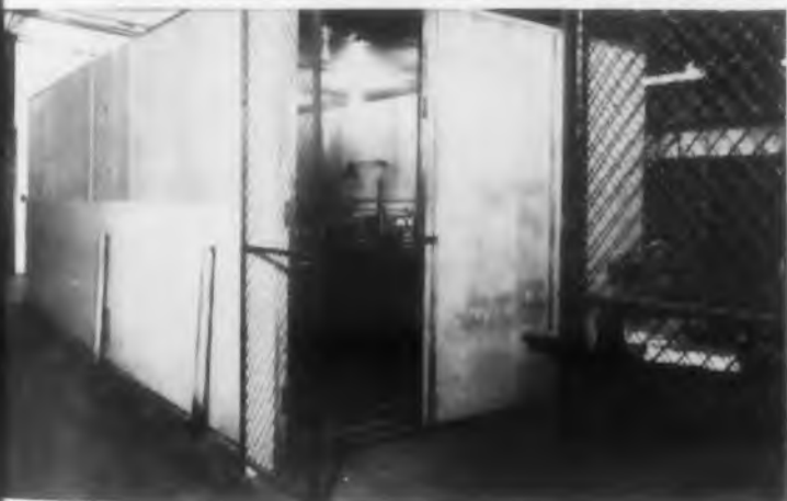
Shielded room, 10' x 20' x 8', designed and manufactured by SHIELDING, INC., Riverton, N. J., for Magnavox Corporation, Ft. Wayne, Ind.
