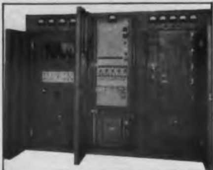
POWER CUBICLE ● CONTROL CUBICLE ● RF CUBICLE TYPE MS WESTINGHOUSE LINEAR AMPLIFIER
