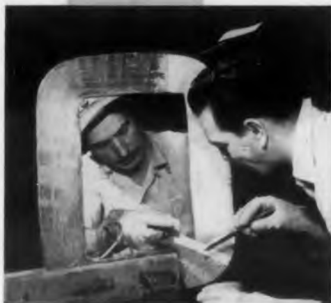
Applying Epon resin sealing compound, formulated by Epoxyllite Corporation, El Monte, California, to a 400-kva transformer winding at Larsen-Hogue Electric Co., Los Angeles, Calif.
