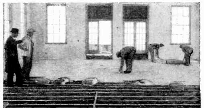
Modern building science has devised packing by which dance floors are made sound proof. Spaces are left between structural parts to prevent bothersome sound-travel beneath the floor. In pursuit of knowledge about the sound-carrying qualities of building materials, the Bureau of Standards makes and breaks numerous houses like the one shown at the left.
