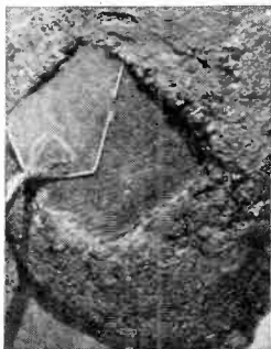
The mixture above shows an excess of cement-sand mortar. The yield of concrete here will be low and probably porous.
