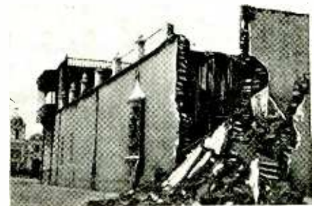
What happens when a heavy rain strikes an unprotected adobe building.
