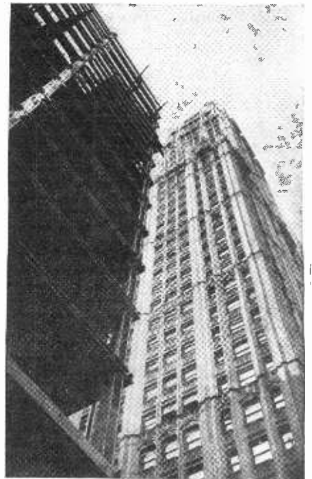
An unusual skyscraper photograph, the camera lens having been pointed skyward—showing the famous Woolworth Building on the right, and a new fifty story neighbor being erected next to it. This photo gives a good idea of the skyscraper's steel frame.
